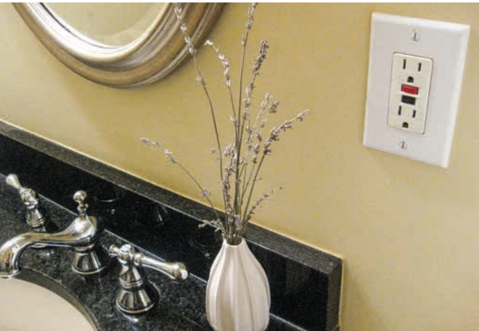
A GFCI should be used in any area where water may come into contact with electrical products, such as the bathroom, kitchen or outdoors.
